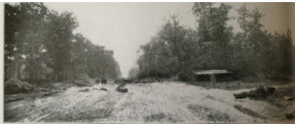
Fiske Terrace at Avenue G and 17th Street looking south showing the opening of 17th Street through woodland; we cut through heavy growth of trees, as may be seen by the trees left standing on either side of the cut. Embankment on line where trees are left standing also shows the quantity of earth we had to haul away (some 100 cubic yards). This view was taken in September, 1905, less than three months after we took title and a year when compared with the following pictures, taken from same position in April of 1906, only ten months after Fiske's name came into our possession.
