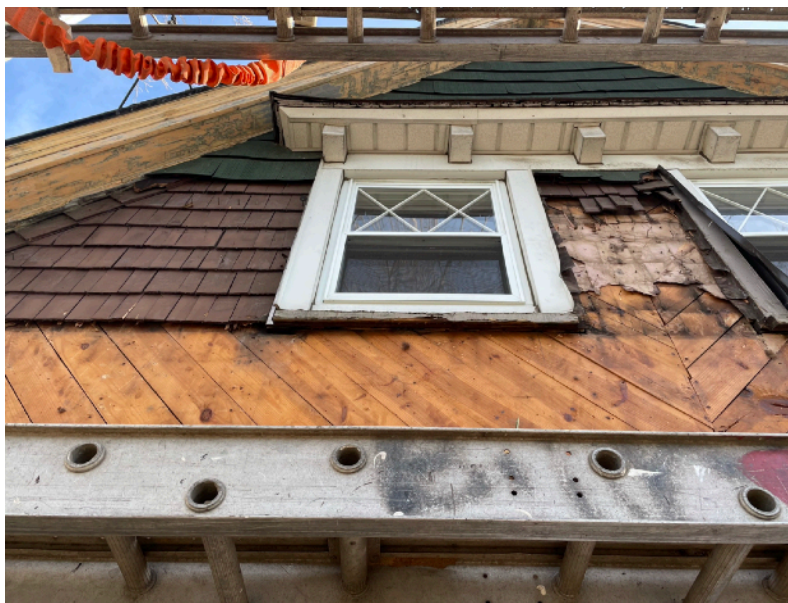
The front gable of 725 Argyle during demolition, with the following layers visible: non-original green asphalt shingles, stained wood original shingles, pink rosin paper,
